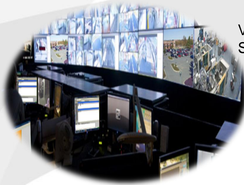
Video Monitoring Systems
